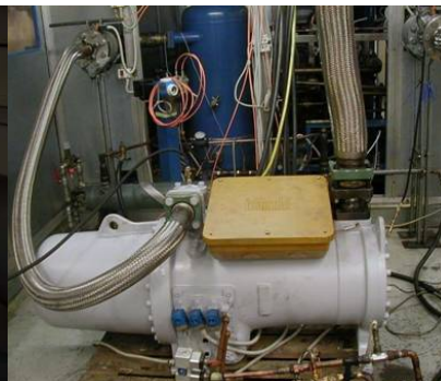
Fig. 7 Refrigeration compressor, Broglia, 2007
