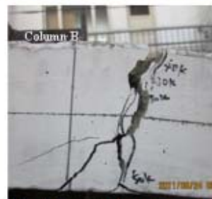
g) Cracks penetrating through slab
