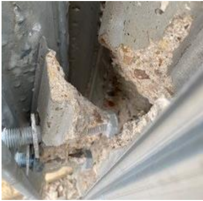
Concrete cone failure.
