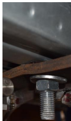
Bolted studs' failure.
