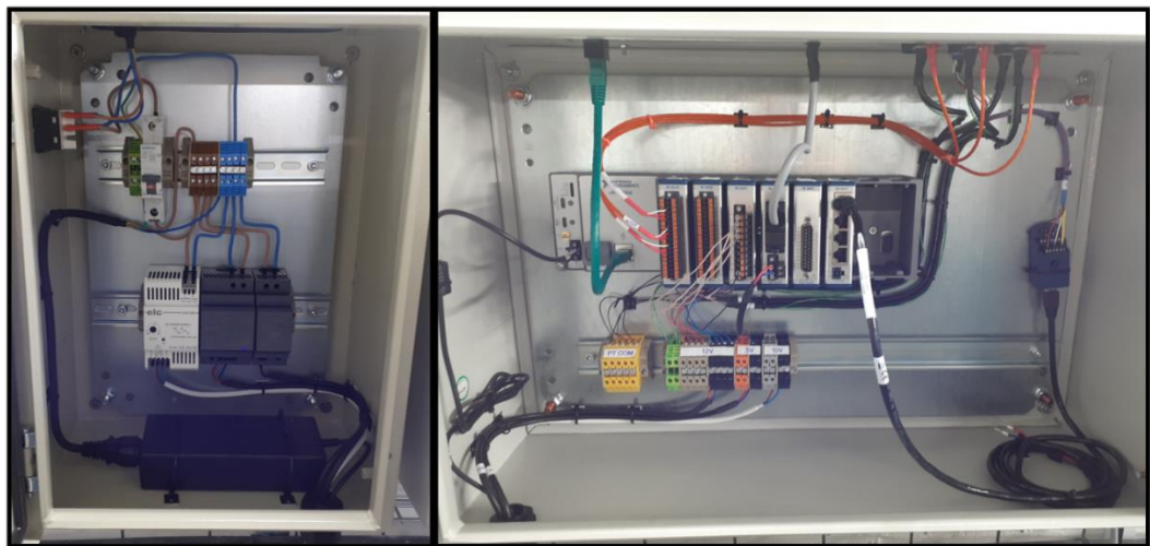
Figure 6.2 DAQ system with Power supply unit
