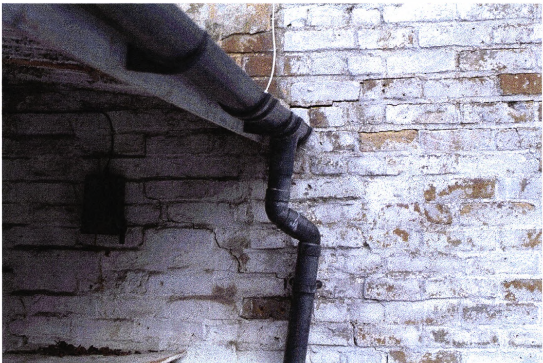
Figure 2.2. The sheltered part of the wall to the left has become soiled, but the paint is intact. On the right, the wall is not roofed. Rain has cleaned the black dust from the pointing, but the coating has failed .
