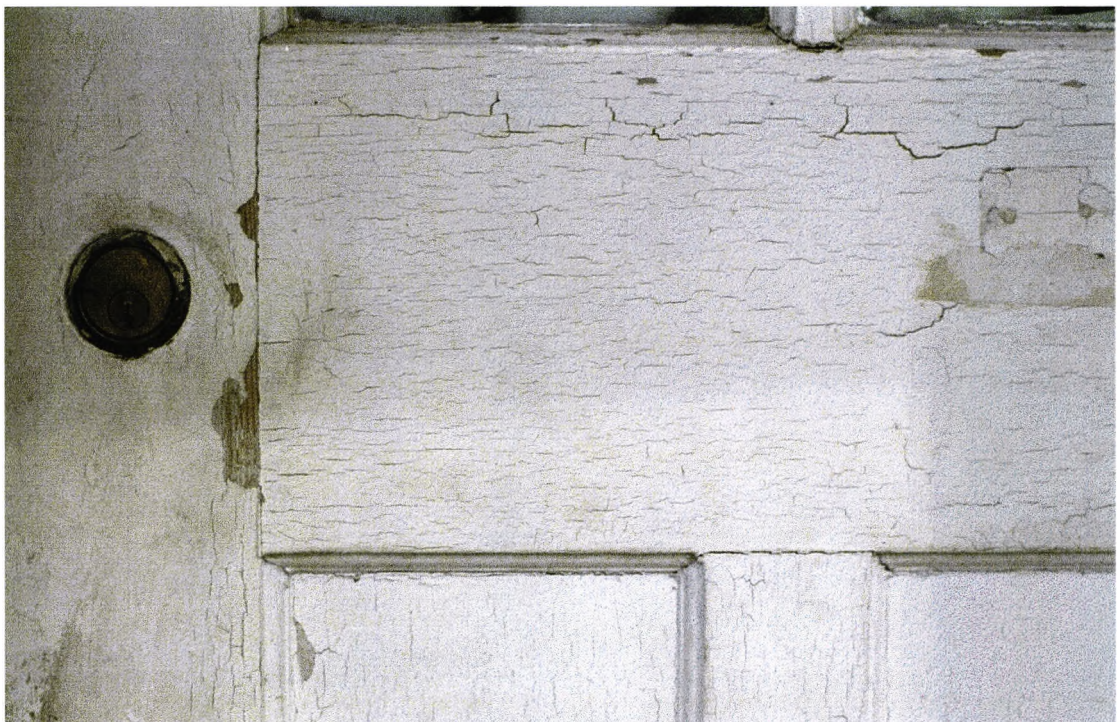
Figure 2.3. Cracking predominately along the grain and direction of brush strokes on this wooden house front door. If the coating had been sprayed onto a substrate with no grain, the cracking would tend to be hexagonal. Some accidental damage can be seen around the lock rose. This could account for the localised flaking.
