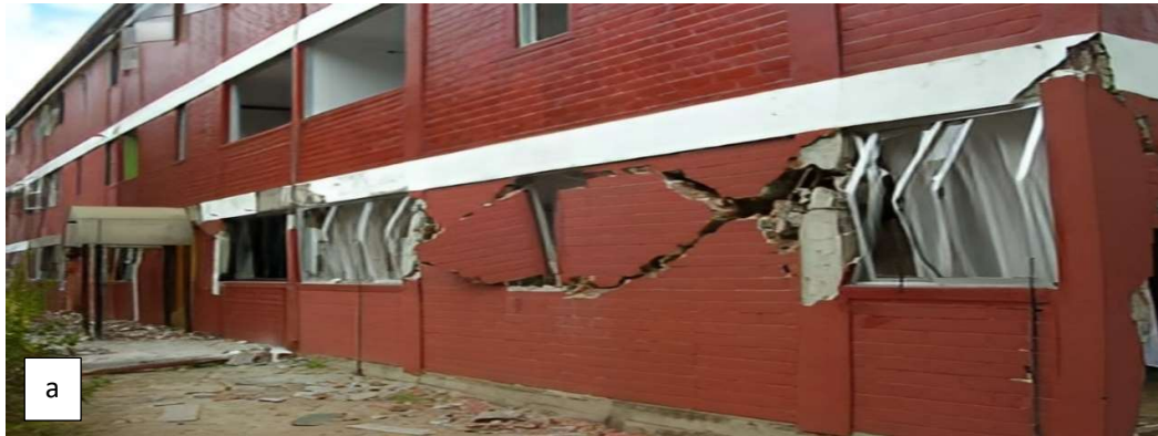
Figure 2.11: In-plane failure earthquake in Izmit, Turkey in 1999 (Casareto et al, 2002)
