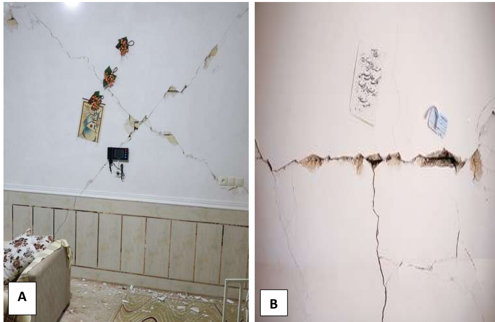
Figure 2.14. Cracks in the wall for out-of-plane and in-plane behaviour (Iran, kokkiloeh, 2021 by Fathi)
