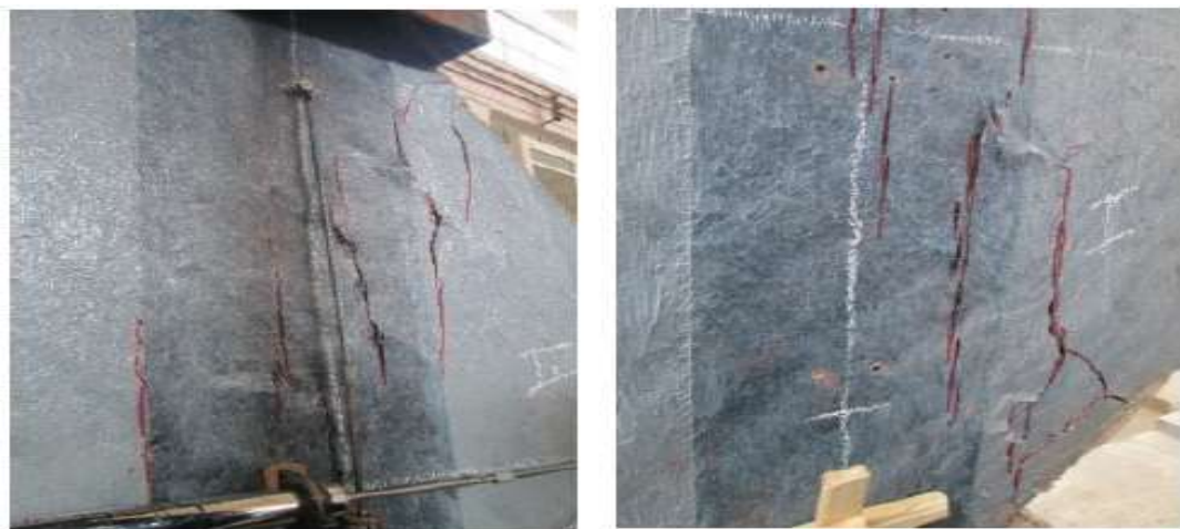
Figure 2.33: Delamination and shear cracking in wall with three parallel diagonals CFRP (El Malyh et al. 2020).
