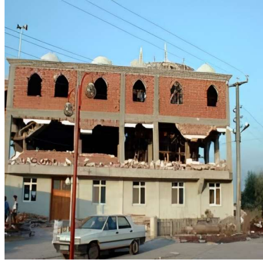
(b) In-plane failure
