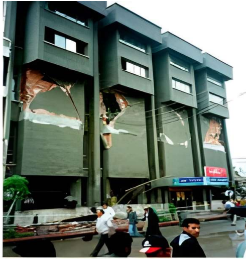
(a) Out-of-plane failure
