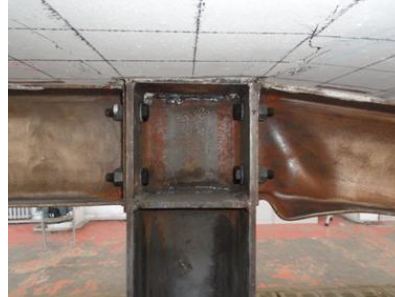
(c) Buckling of beam by column B
