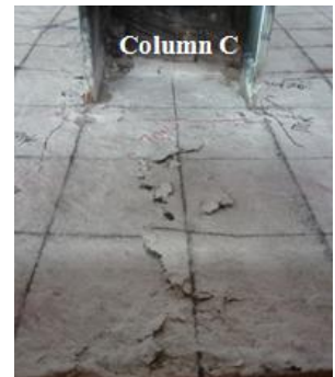
(e) Crush of concrete
