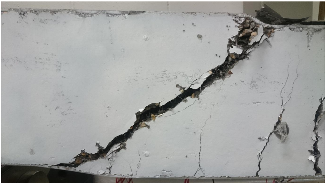
Figure 5.49. Concrete shear crack view for SCB6
