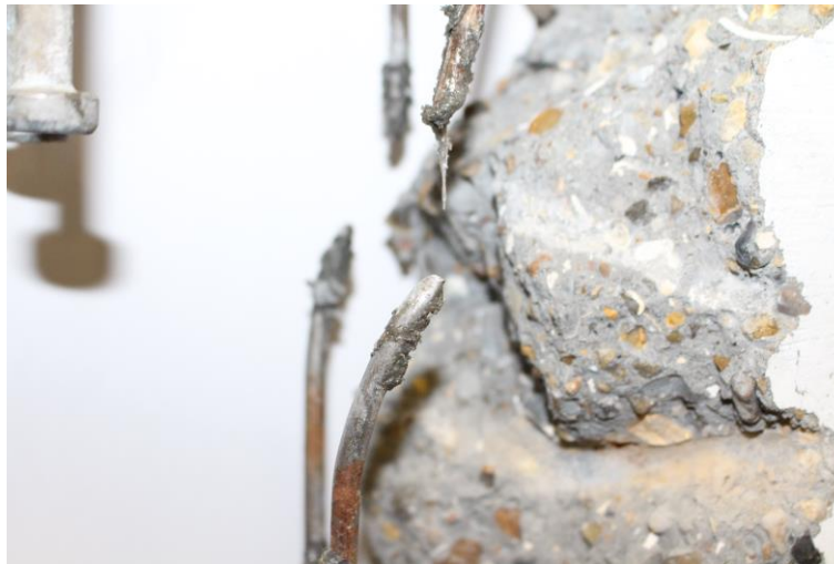
Figure 5.33. Fractured tie bar in SCB4
