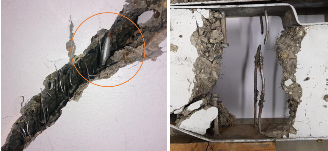
Figure 5.19. Fractured tie bars crossing C4
