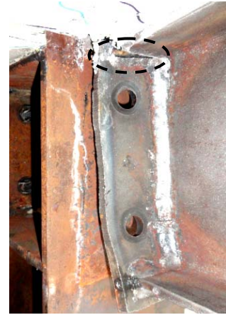
(b)Fracture of welding seam
