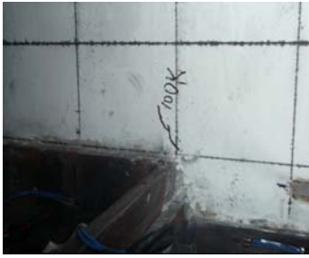
(a) First crack on slab
