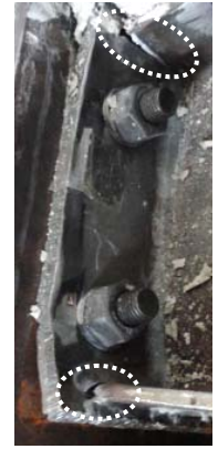
(c)Fracture of welding seam
