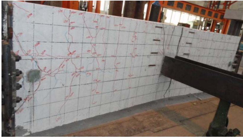
(a)Cracking pattern at top of slab
