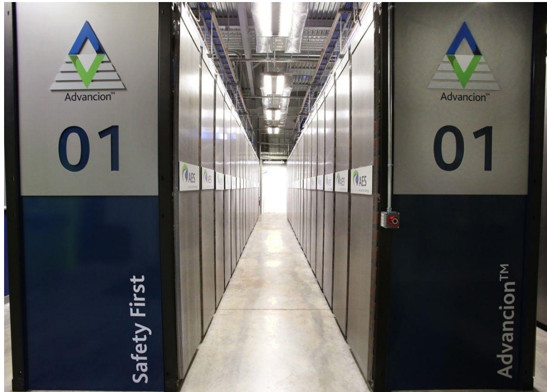
Figure 2.3. Grid-scale battery storage array in Kilroot, Ireland
